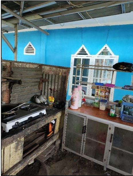
Figure 3. Condition of the kitchen and food storage areas at the food stalls in Alam Barajo Terminal, Jambi City.
